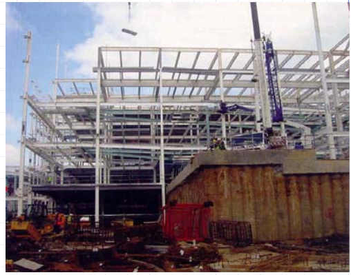
Construction of a multi-storey building, system of primary and secondary beams is visible
